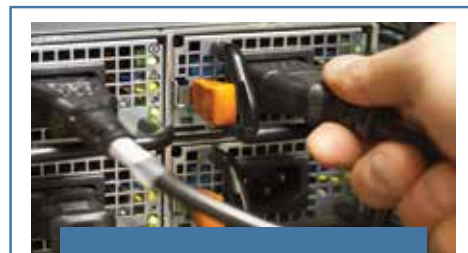
Power Supply Units
